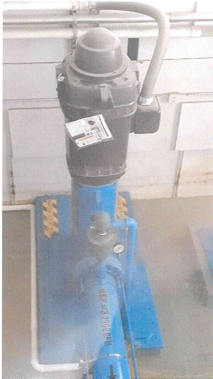
High Service Pump No. 3
