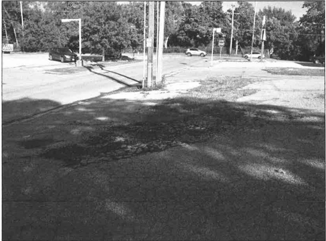
307 NE 58 th Street – looking east – deterioration of parking surface, driveway
