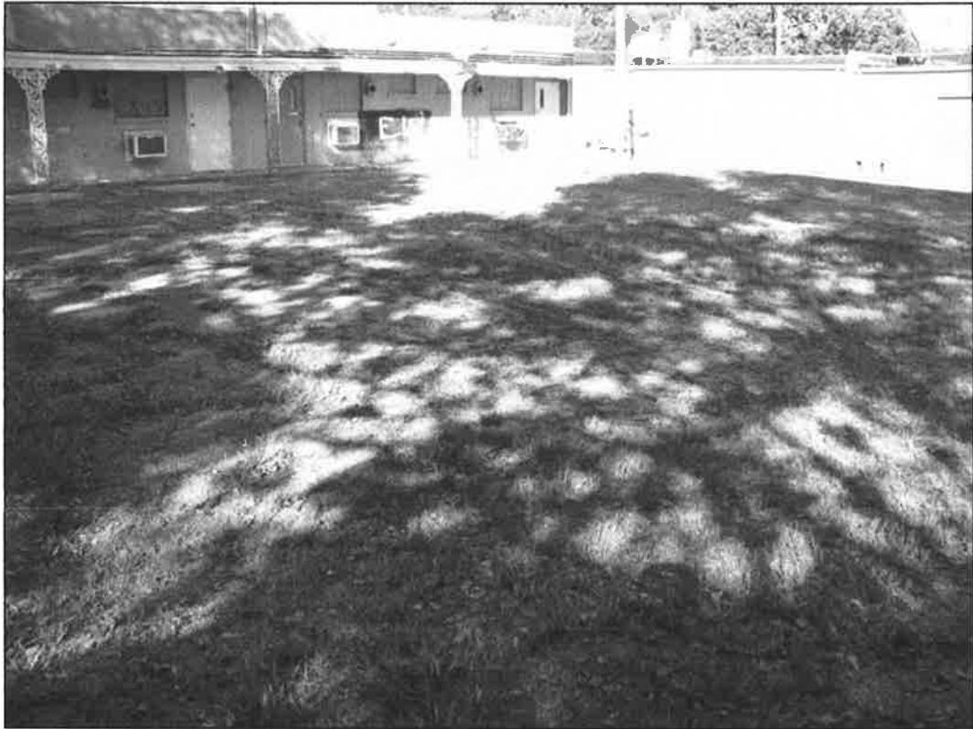
307 NE 58 th Street – looking northeast – deterioration of parking surface
