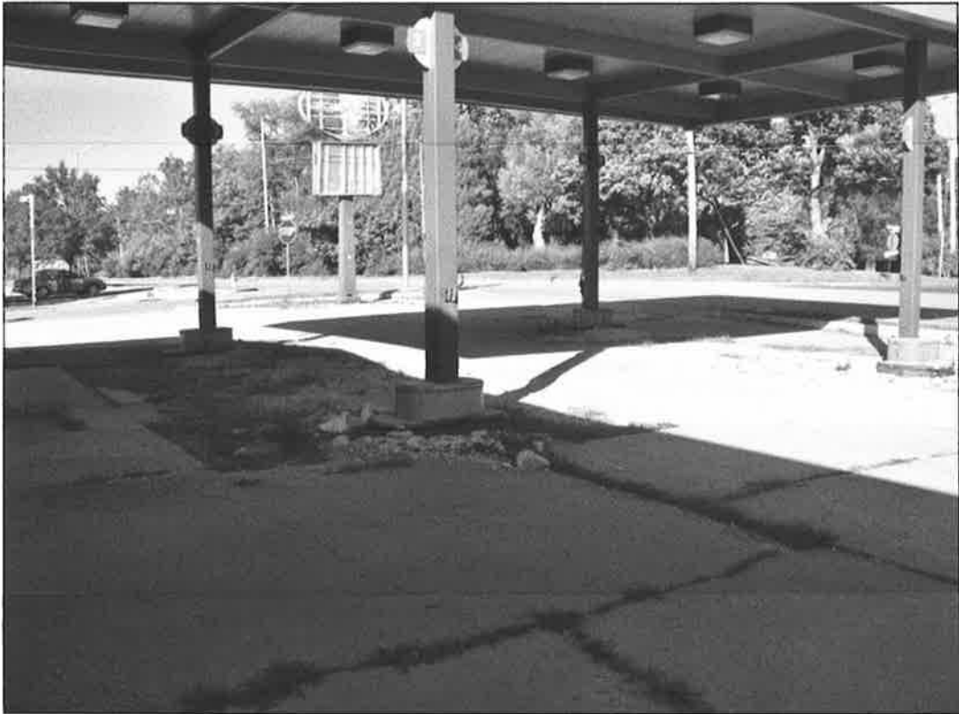
5720 N. Oak Trafficway – looking northeast – deterioration of pavement
