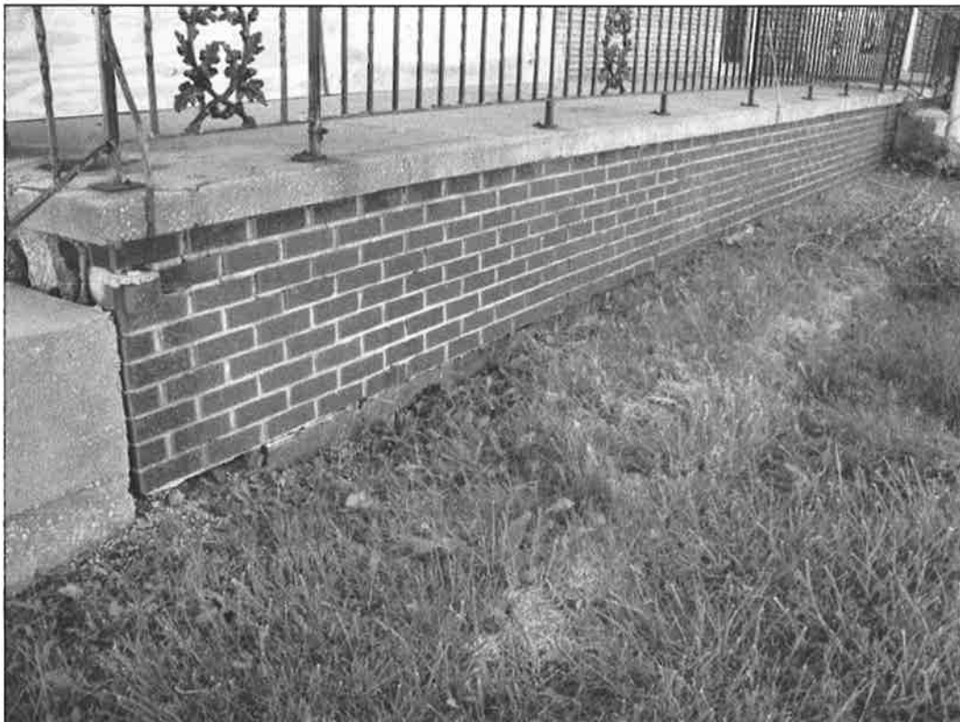
307 NE 58 th Street – looking southwest – deterioration of masonry veneer, foundation
