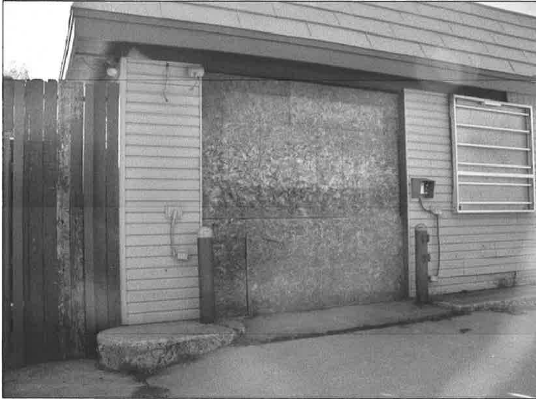
5720 N. Oak Trafficway – looking west – deterioration of door, siding, signage; failure of finishes
