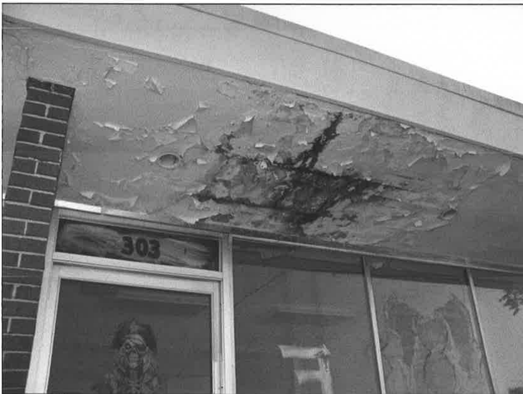
307 NE 58 th Street – looking south – deterioration of soffit (due to leaking roof)
