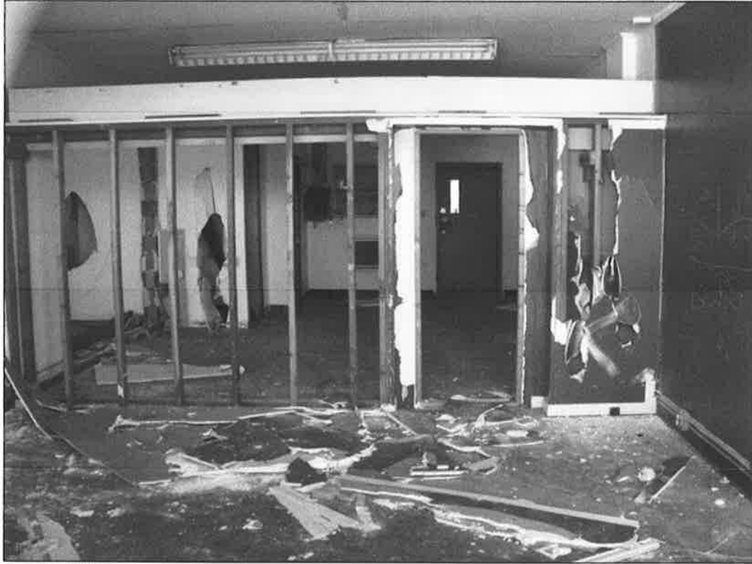
307 NE 58 th Street – looking south – deterioration of interior finishes, windows; outdated building systems
