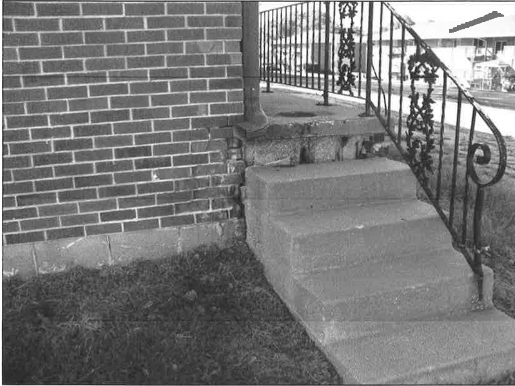
307 NE 58 th Street – looking west – deterioration of masonry veneer, steps; failure of finishes
