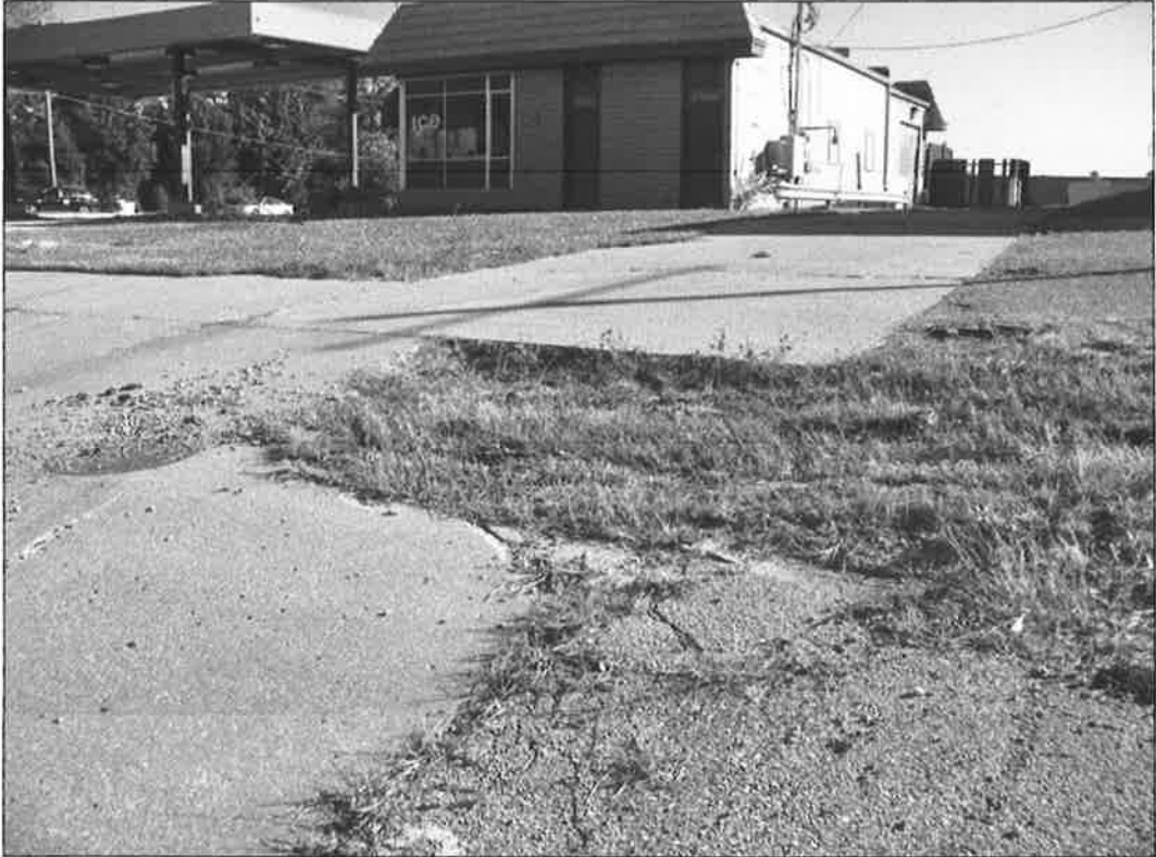
5720 N. Oak Trafficway – looking south – deterioration of driveway
