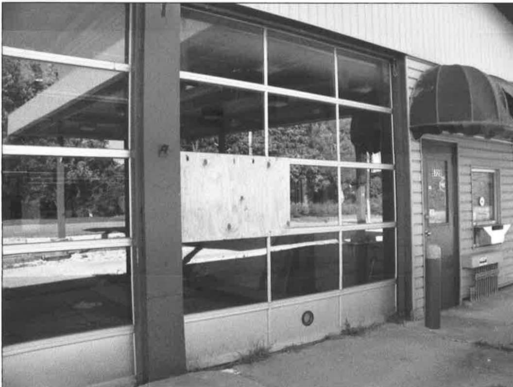
5720 N. Oak Trafficway – looking west – deterioration of door, awning; failure of finishes
