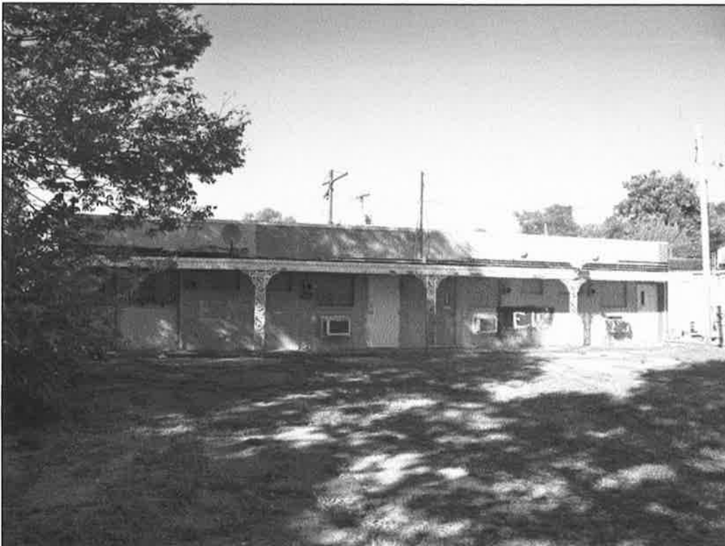
307 NE 58 th Street – looking north – deterioration of roof, windows, doors, mechanical systems
