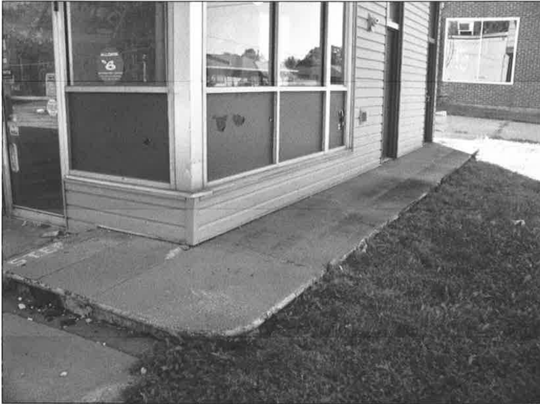
5720 N. Oak Trafficway – looking west – failure of finishes
