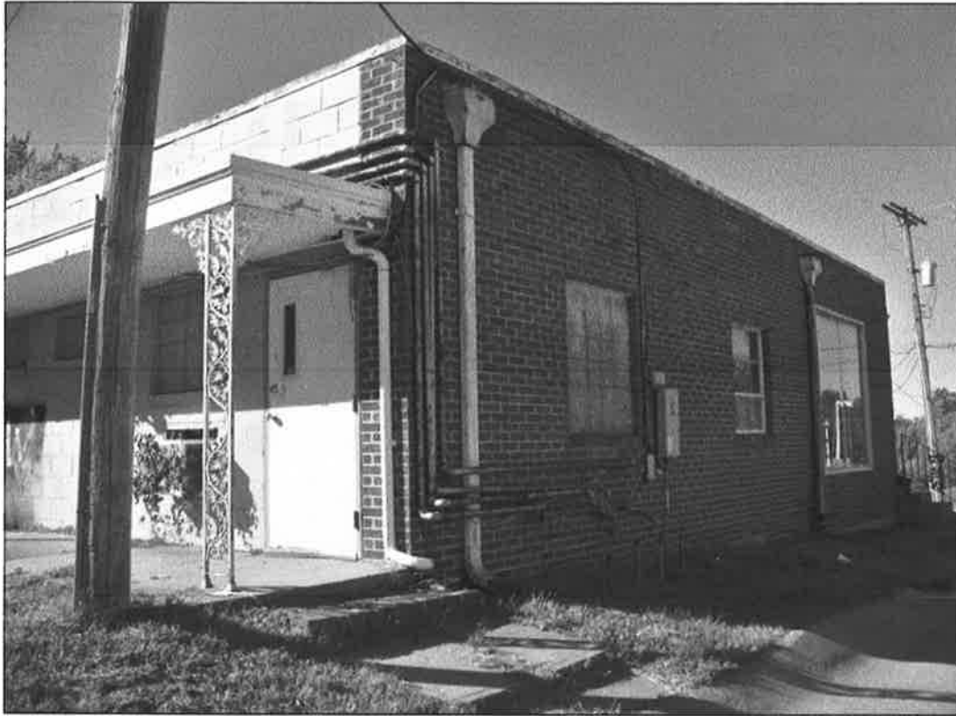
307 NE 58 th Street – looking northwest – deterioration of windows, doors, mechanical systems, downspouts
