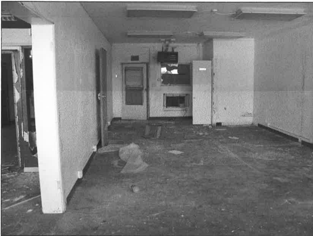
307 NE 58 th Street – looking south – deterioration of interior finishes, windows, doors; outdated building systems
