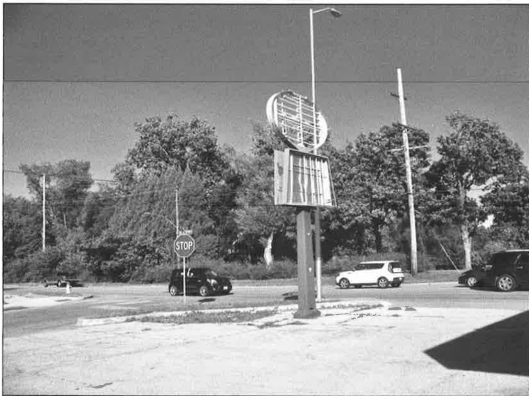
5720 N. Oak Trafficway – looking northeast – deterioration of sign, pavement; failure of finishes
