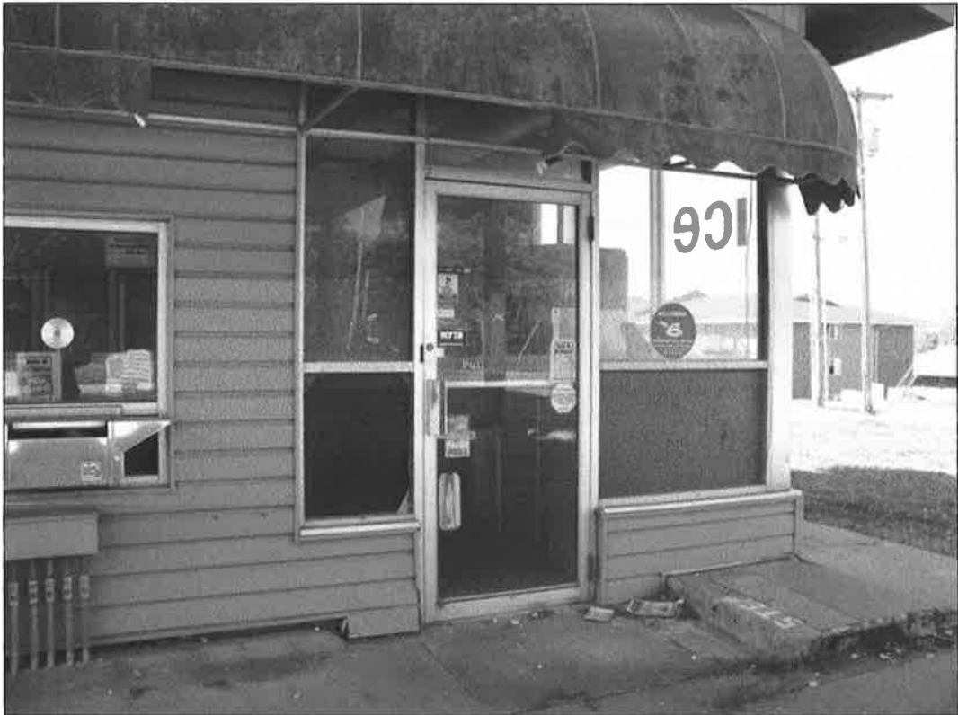
5720 N. Oak Trafficway – looking northwest – deterioration of awning, sidewalk; failure of finishes
