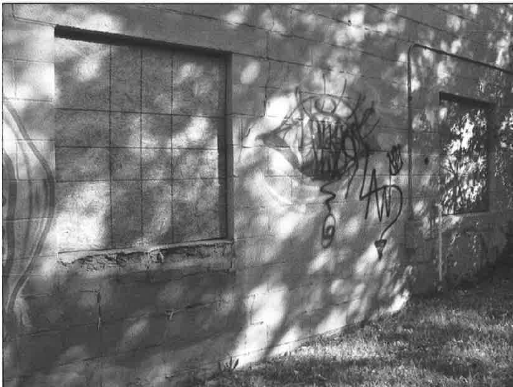
307 NE 58 th Street – looking east – cracked and spalling masonry wall; deterioration of window; failed finishes
