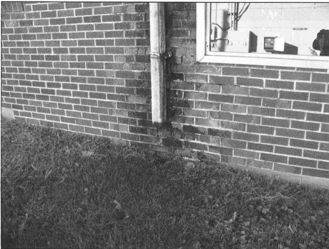
307 NE 58 th Street – looking west – deterioration of masonry, downspout
