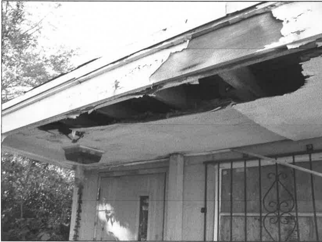
307 NE 58 th Street – looking north – deterioration of fascia, soffit, window, roof coping; failure of finishes
