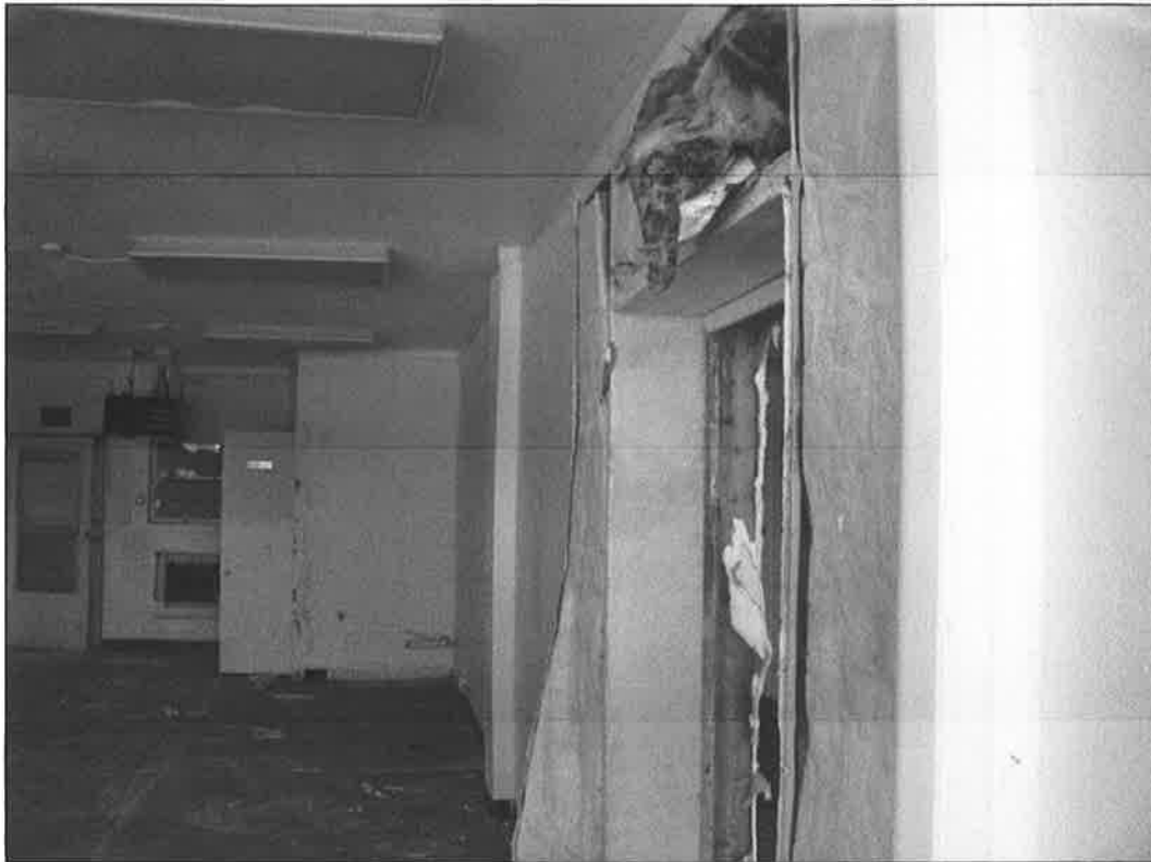
307 NE 58 th Street – looking south – water damage from leaking roof, mold
