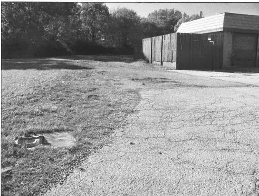
Parcel No. 13909000500600 – looking west – deterioration of driveway
