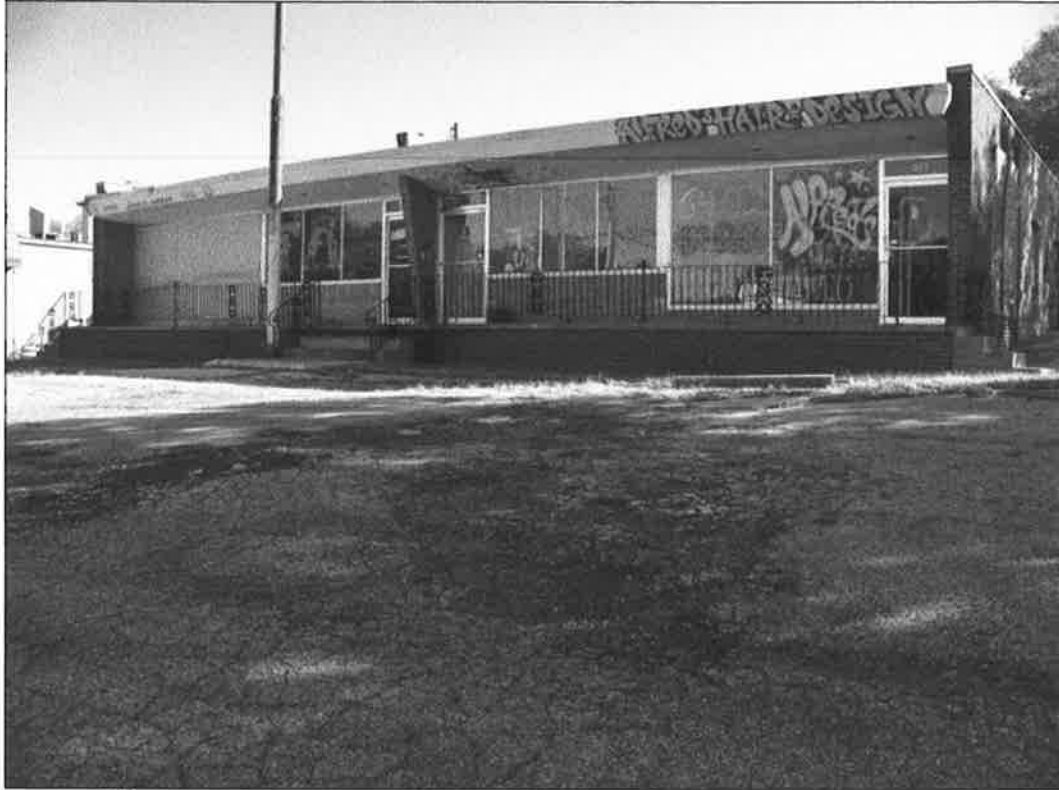
307 NE 58 th Street – looking south – deterioration of windows, parking surface
