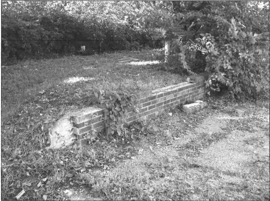
307 NE 58 th Street – looking west – deterioration of masonry wall, parking surface
